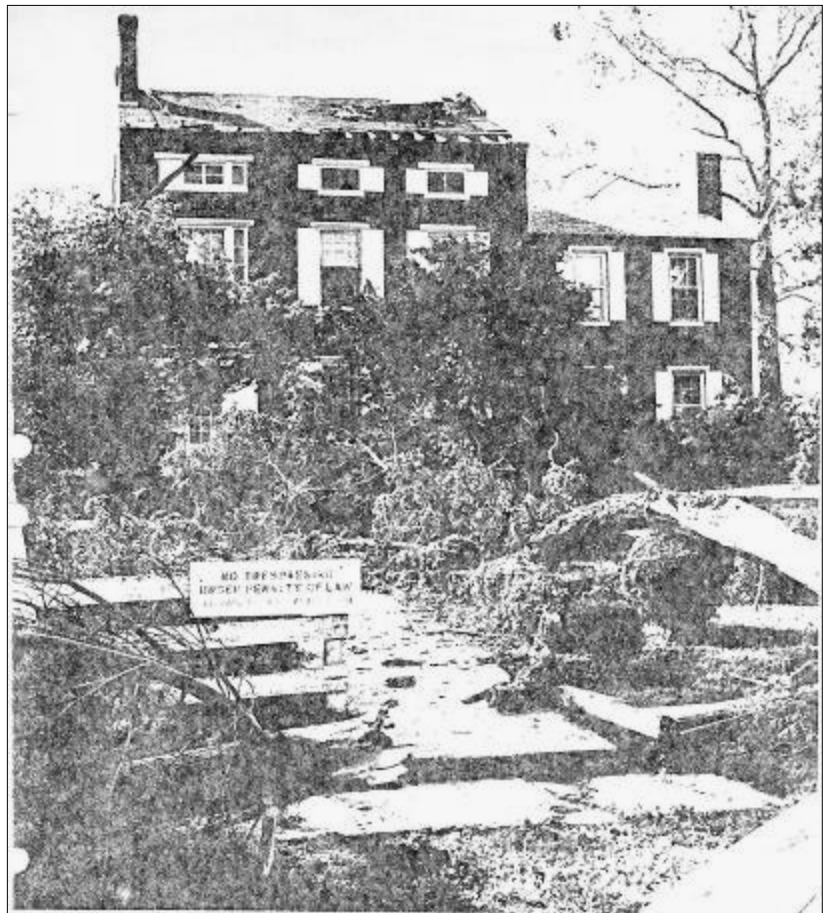
Tornado damage to Needwood Mansion 1968. Trees blown over during the tornado punched a large hole in the roof and knocked down chimneys.
